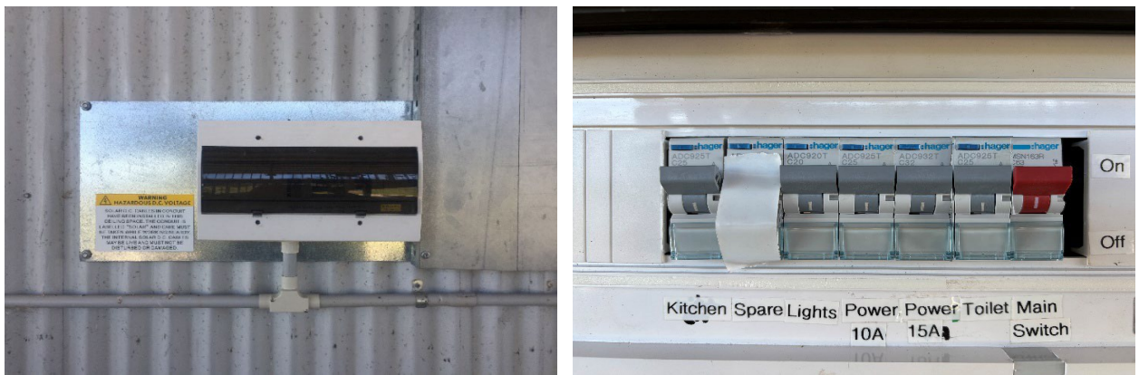
Fig 5. Member Accessible Switchboard
